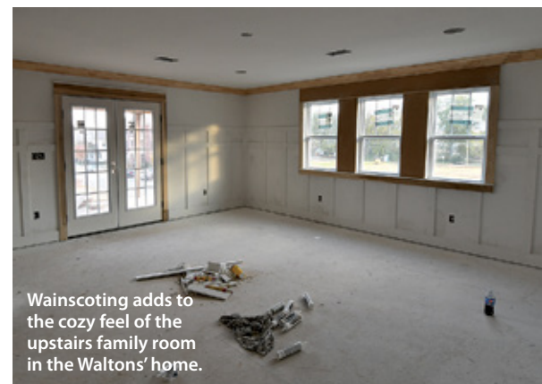
Mitch and Terri Walton are eagerly awaiting the completion of their new home in Legacy Park.
